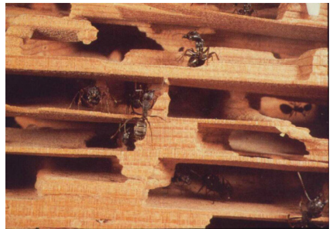
Fig. 7. Carpenter ant tunnels. 5
